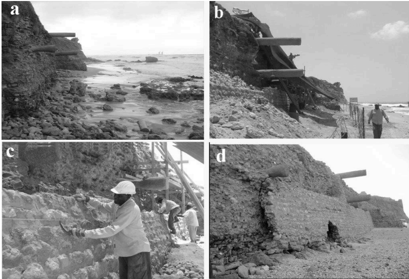
Fig. 14 - Ashkelon sea wall under reconstruction works: a) before works, b, c) a protective layer is being built on the wall face, d) the protective layer underwent erosion by the storm waves (E.G.).
